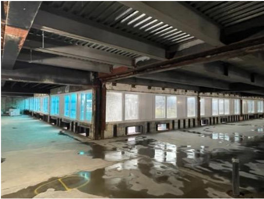
All windows have been installed - view of the Studio Bedroom Wings for independent & assisted living units
