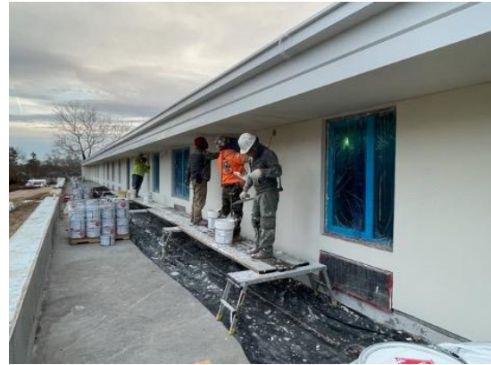
Stucco being applied to the outside of the independent Living One-Bedroom Apartments, each with a Terrace
