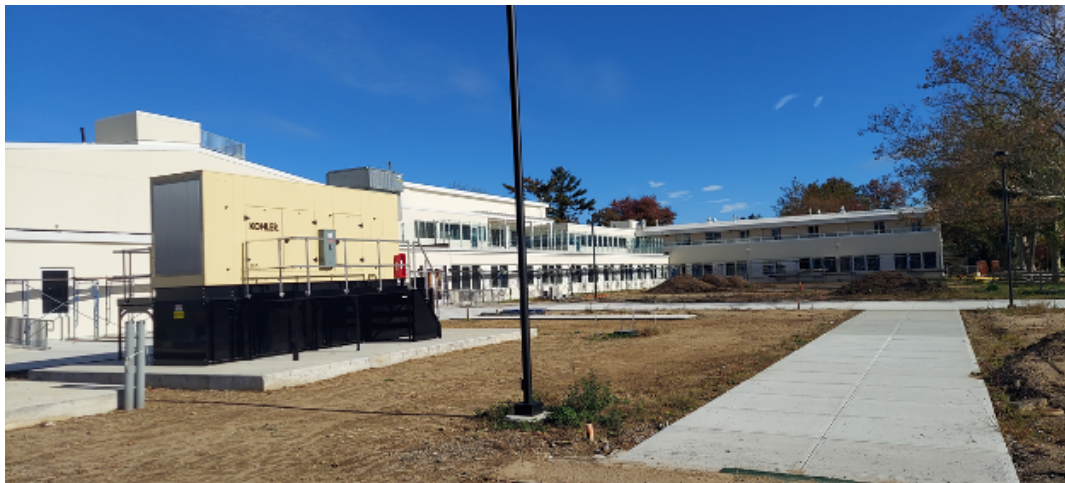
Rear View of the facility & generator
