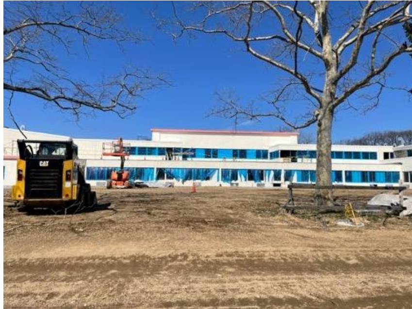
View of side façade with well advanced stucco work and installed windows
