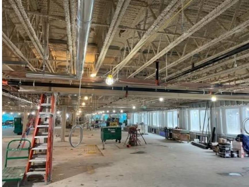
Interior east wing with spray fireproofing and sprinkler piping; note installed windows
